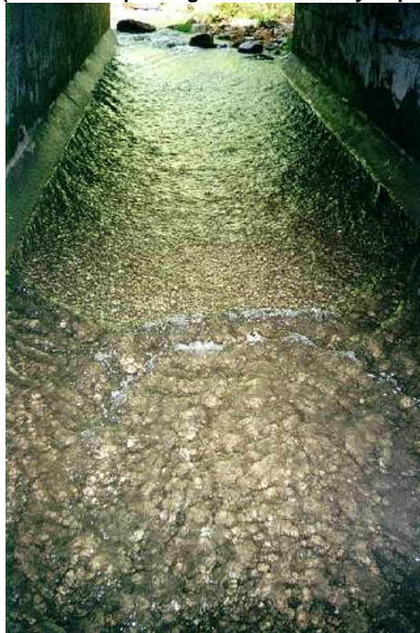
Figure 6-3. Shallow Depth of Supercritical Flow in Culvert (From Road Engineering Journal, Transafety, Inc.)
