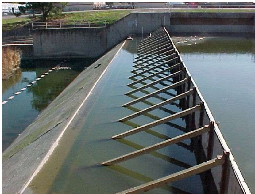
Figure 6-1. Excessive Elevation Drop (Alamitos Drop Structure, Guadalupe River)
